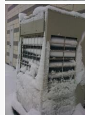
Freezing issues of air-source heat pumps
